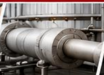
INDUSTRIAL (CRYOGENIC INSULATION)
